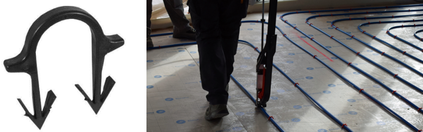
FIGURE 6: TACKER ON THE LEFT AND INSTALLATION OF THE UNDERFLOOR HEATING ON THE RIGHT
