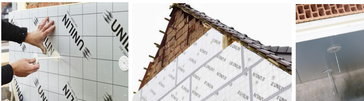
FIGURE 8: PLACING THE PLUGS THROUGH THE INSULATION AFTER DRILLING, THE TAPE IS VISIBLE ON THE MIDDLE PICTURE, THE ANCHOR ON THE RIGHT
