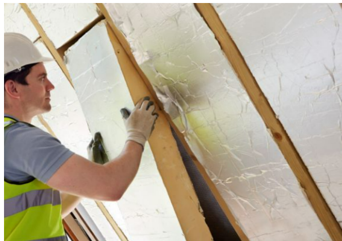
FIGURE 20: PU BOARDS BETWEEN THE RAFTERS
