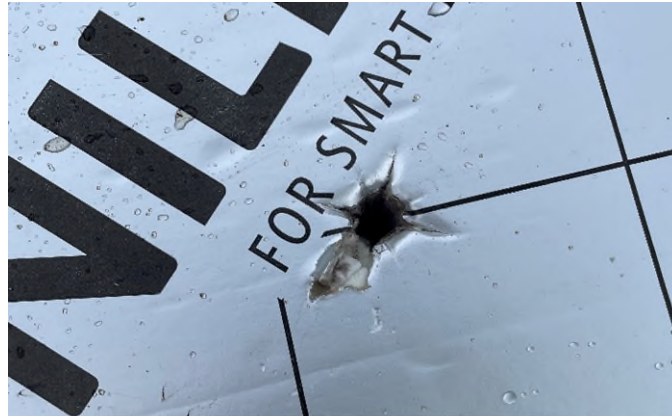
FIGURE 12: DAMAGE TO THE INSULATION BOARD AFTER REMOVAL MECHANICAL FASTENING MATERIALS
