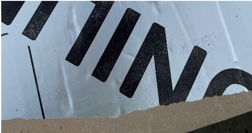
FIGURE 9: DAMAGE TO THE FACER, SEEN AT THE BOTTOM OF THE FIGURE
